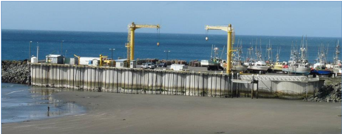
Source: Port of Port Orford, June 2012. Notes: 1. See boats and cranes on dock itself. 2. Shoaling of the harbor as seen at minus tide, showing dock sheet pile construction and aging high-capacity cranes used to launch and retrieve vessels.
